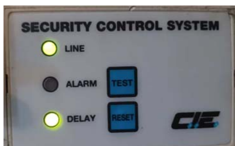
SECURITY CONTROL SYSTEM
